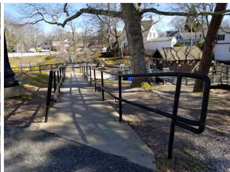
Non-Compliant H/C Ramp
