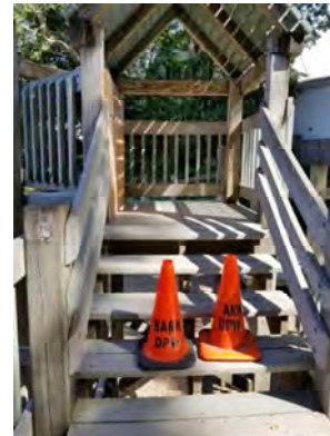
Steps need repair
